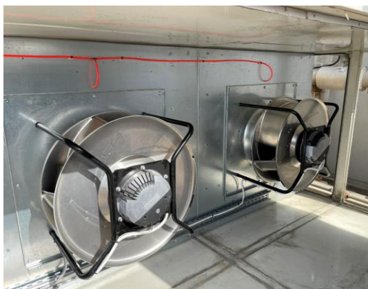
Fig. 2: A total of 26 RadiPac were installed as FanGrid in both the supply and exhaust air section of the four AHUs.
